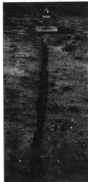
Figure 5: Item #12 Settling Trench
