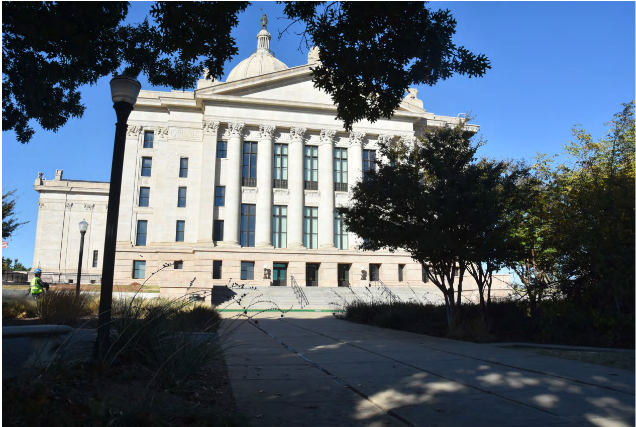
Top: The east side of the Capitol is shrouded in a cocoon of fabric in October 2017, while workers clean and repair the building's exterior.
